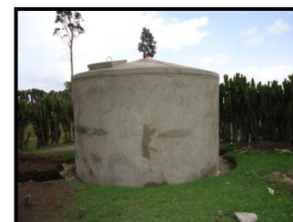
27,000 L reservoir supplying 3 villages
