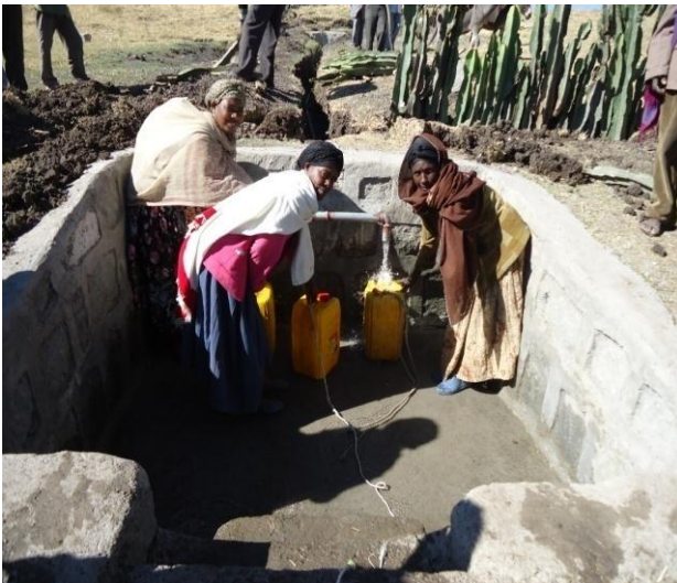
New capped spring at Fencha Village
